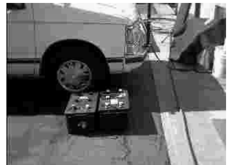
Steve and Imelda's van with two of the six batteries used for power (600kg worth!).
