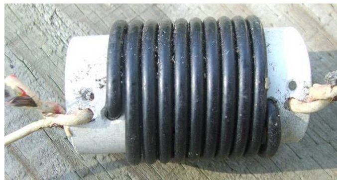
Photo 3 There were wires coming out of the holes and they were soldered onto the cable ends!
