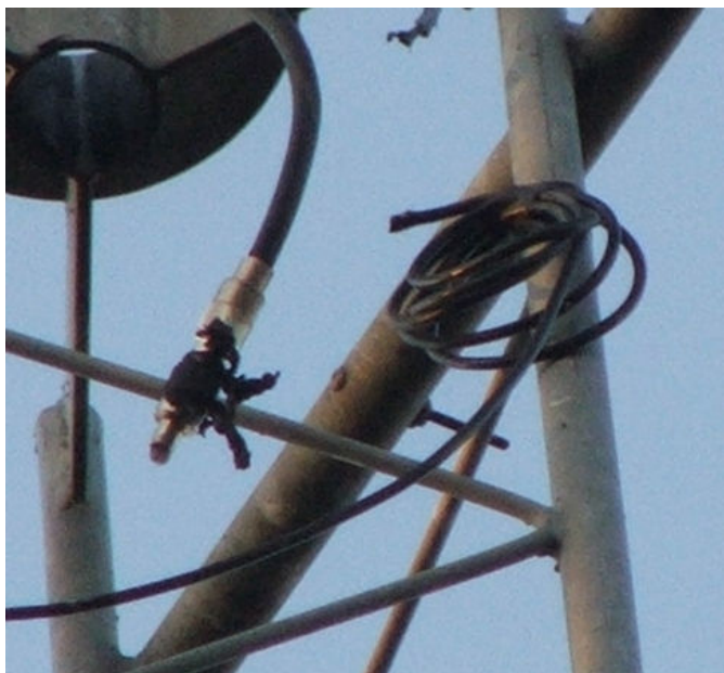
Photo 1 Can you spot to fault? The cable has been cut and the waterproof tape stripped off at the top of the tower.
